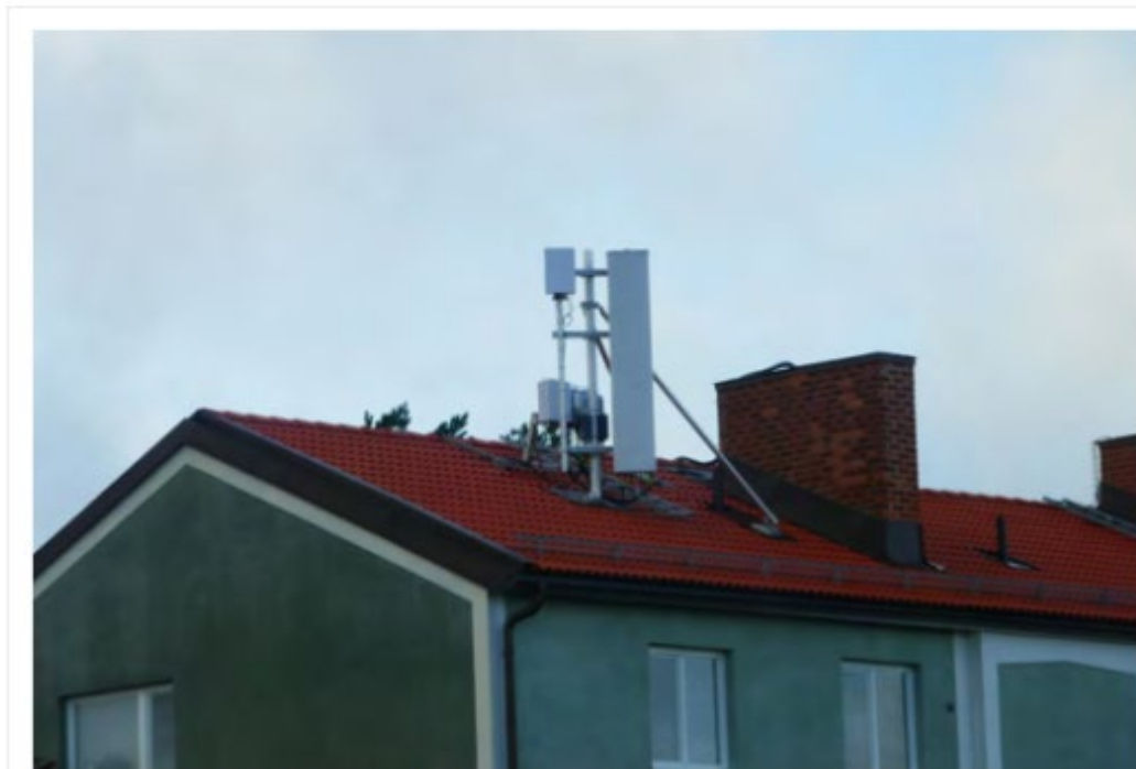
Figure 2: 5G base station on the roof of a three floor building located 60 meters from the study apartment
