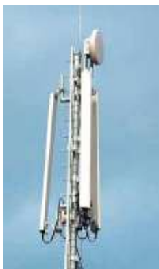
Typical mobile phone base station with three sector antennas and a microwave radio
