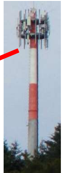
12 OCT 2021 Mobile phone base station and BOS digital radio above St. Blasien
