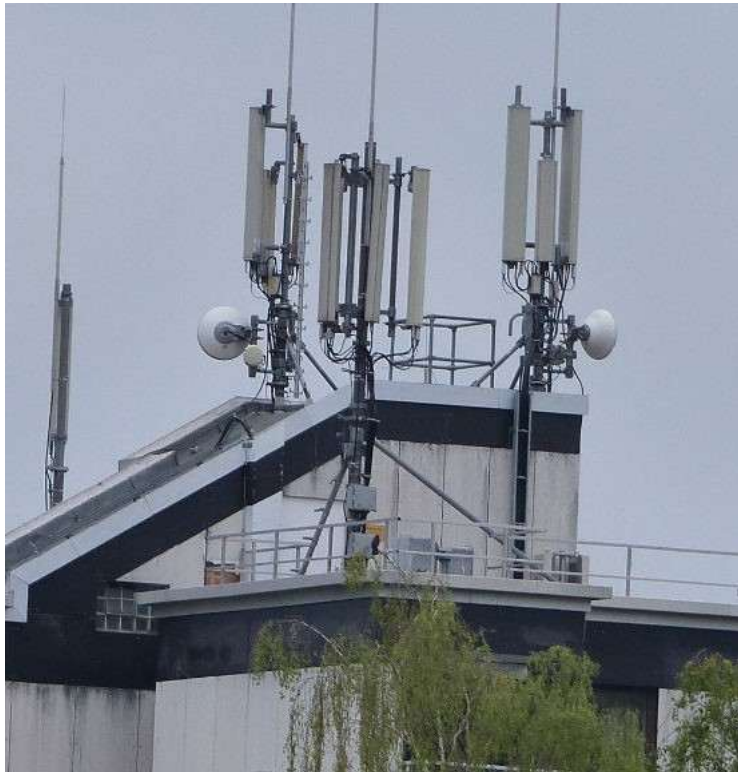
Mobile phone base station at Hunrodstraße
