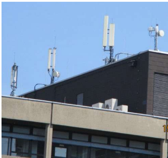
Mobile phone base station on the rooftop of the Institute of Chemistry. Site certificate from December 23, 2019: installation height 31 m (100 ft), 9 sector antennas
