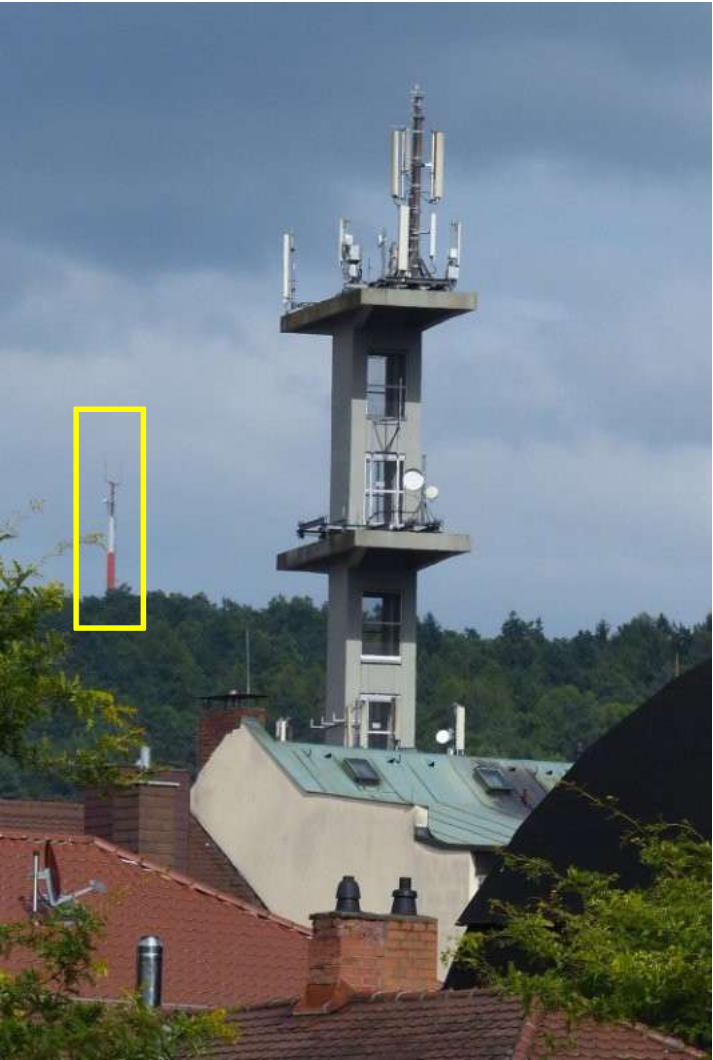
Mobile phone base station No. 660012, near Theaterplatz (installation height 30–48 m / 98–157 ft) and TETRA base station at the eastern hill. 09 NOV 2009: 21 sector antennas 18 APR 2016: 27 sector antennas 11 SEP 2018: 33 sector antennas
